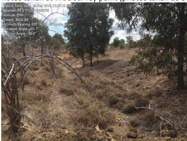
Photo looking north (upstream) from WB6 showing channel depression with no defined banks
